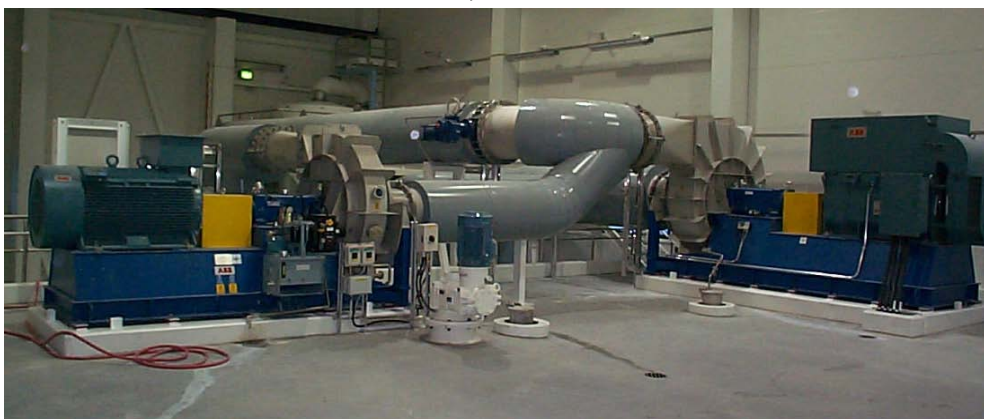
MVR fans in an EPCON evaporator
