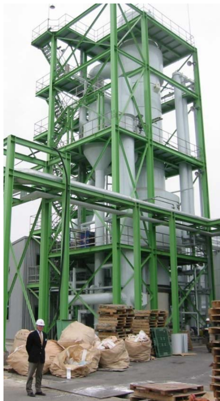
Combined falling film and forced circulation MVR evaporator.
