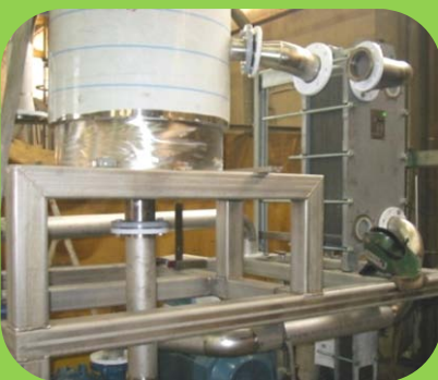
Assembly of EPCOVAP-MVR-4
