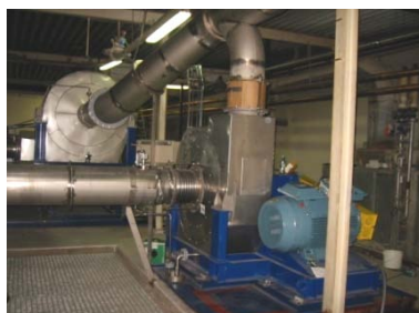
MVR fans installed at the factory.
